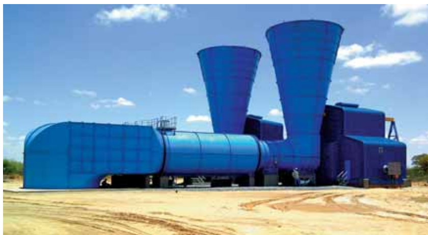
New centrifugal fan installation serving the extension of the Morupule Colliery in Botswana. The fans have been manufactured by Howden fans and the installation is by Howden Projects
