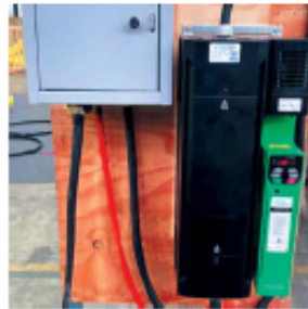
Picture 9. Variable Speed Drive Control
