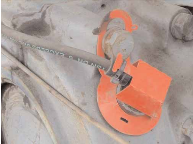
Figure 5: Original bearing temperature sensor
