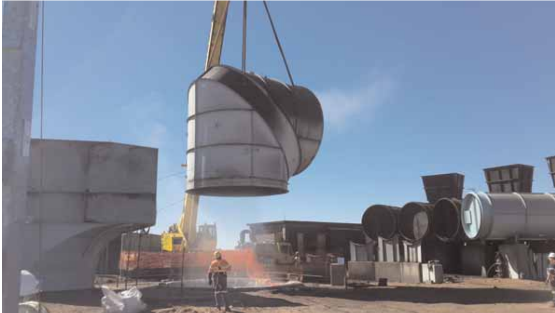
The new shaft top being lowered into place over the mouth of Black Rock mine's 500 m deep main vent shaft.
