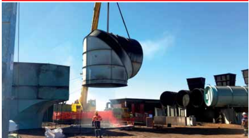
ACTOM Mechanical Equipment mine vent retrofit project at Black Rock manganese mine. See page 30
