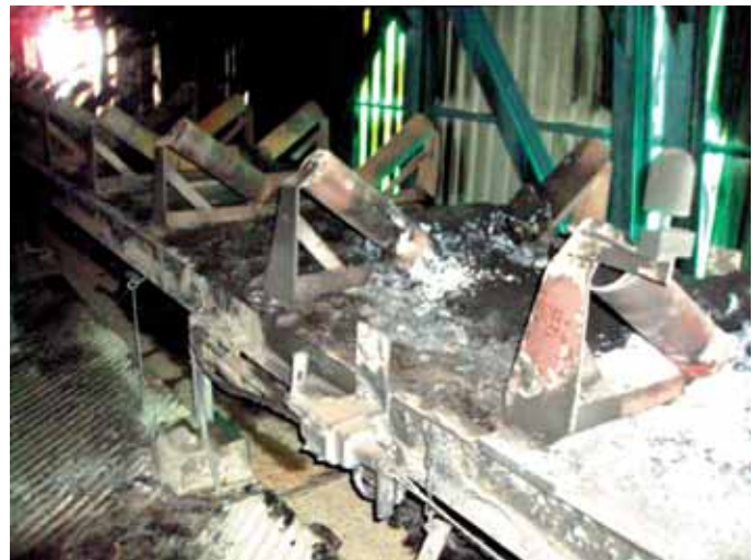
Figure 15: Damaged idler section
