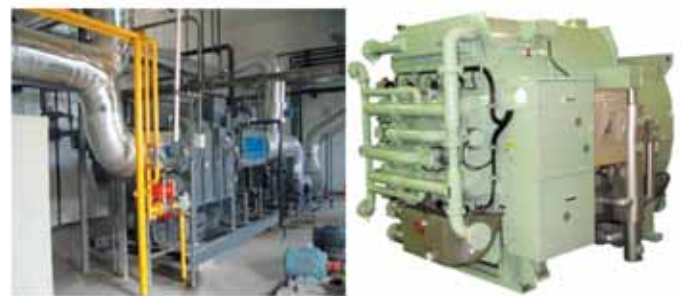
Figure 23: Absorption and Adsorption chillers
