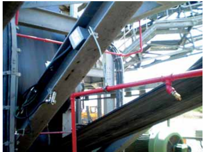
Figure 7: Temperature scanner mounted on conveyor structure
