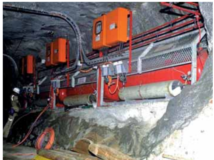
Figure 12: A three tank CAF system installed underground
