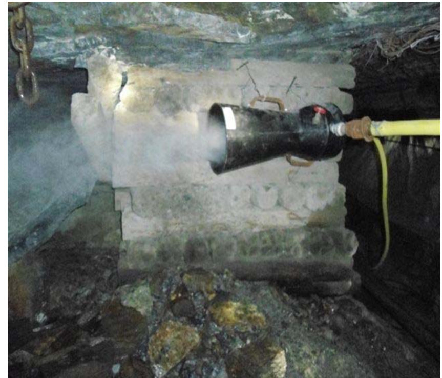
One of the underground installations
