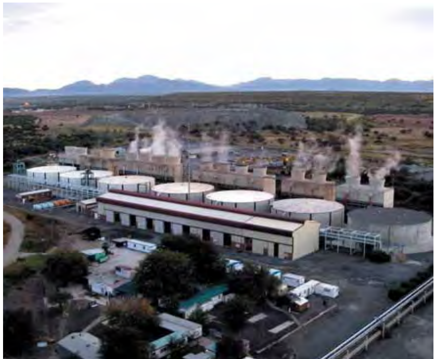
Photo taken by Louis Nel. Refrigeration plant for deep platinum mining
