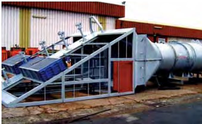
Figure 5. Bank of cooling coils
